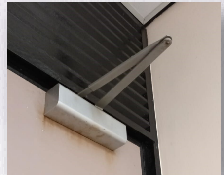
Figure 1. Door drum/ closer in the isolation room
